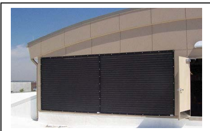
Louver Intake Filters
