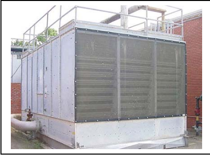
Cooling Tower Filters
