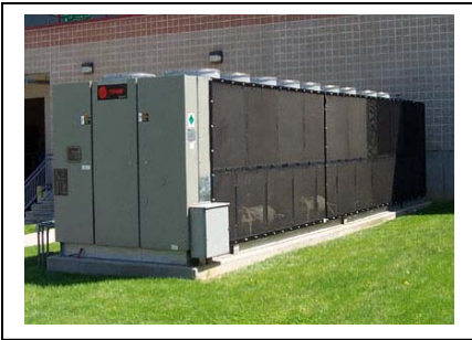
Chiller Coil Filters
