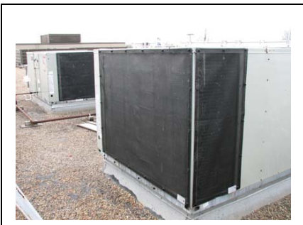
Rooftop Unit Filters
