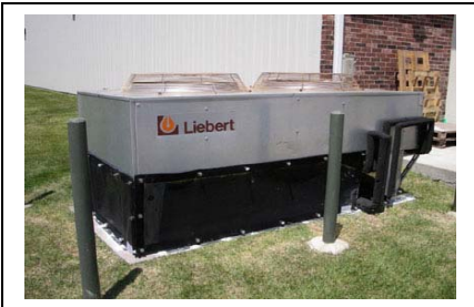
Dry Cooler Filters
