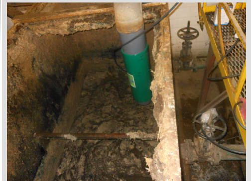
Edge-800-PF-4X Installed with Tank Empty
