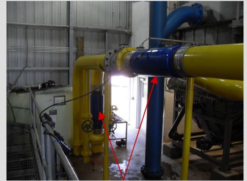
Two 12" EDGE Installed in DAF Feed Lines
