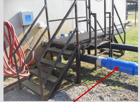
6" EDGE Installed in 1 of 2 DAF Feed Lines
