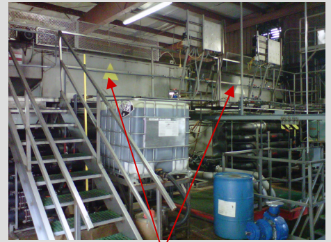
Twin DAF Clarifiers
